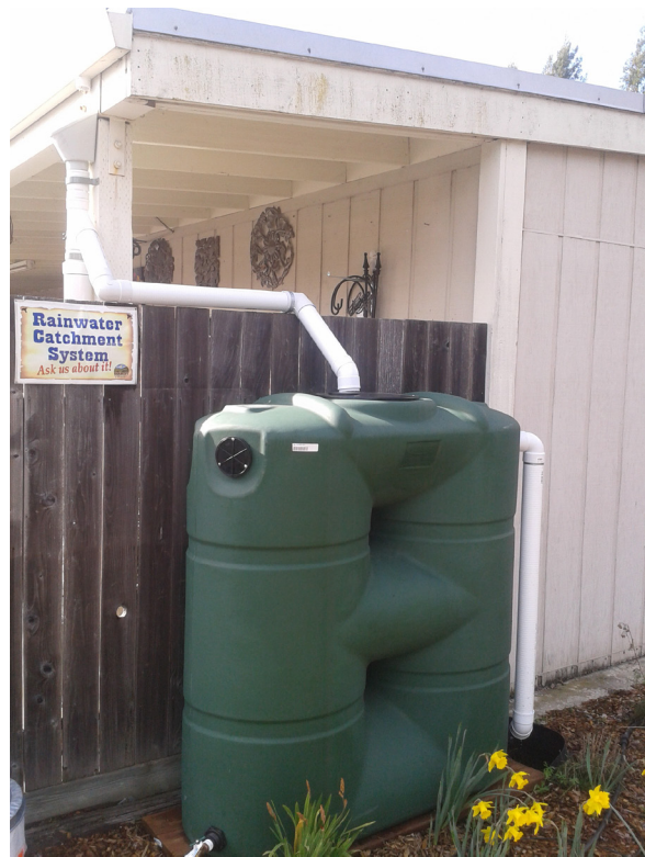
265 Gallon Slimline Tank Installed at Harmony Farm Supply
